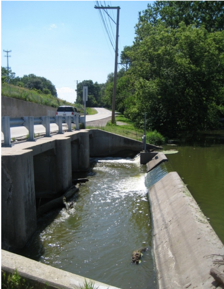
Former Churchill Woods dam (E. Branch RM 18.6 at Crescent Rd. (Note: dam wall removed in February
