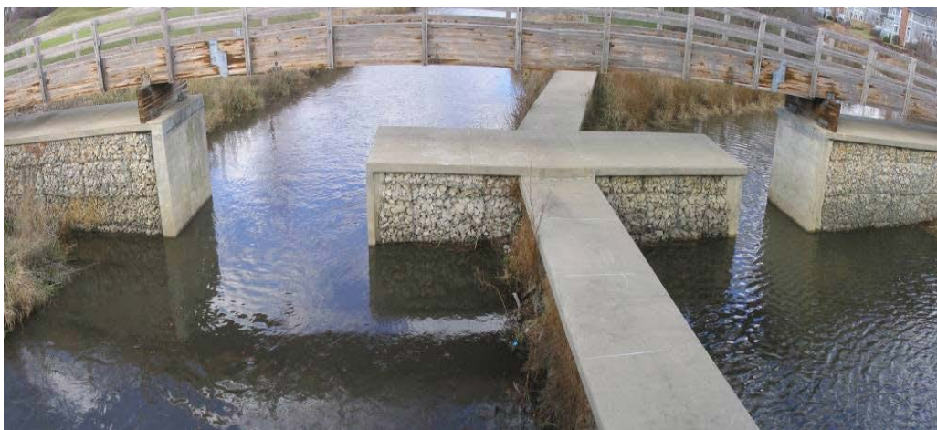
Prentiss Creek stormwater control dam on E. Branch DuPage R. at the Seven Bridges Golf Club.
