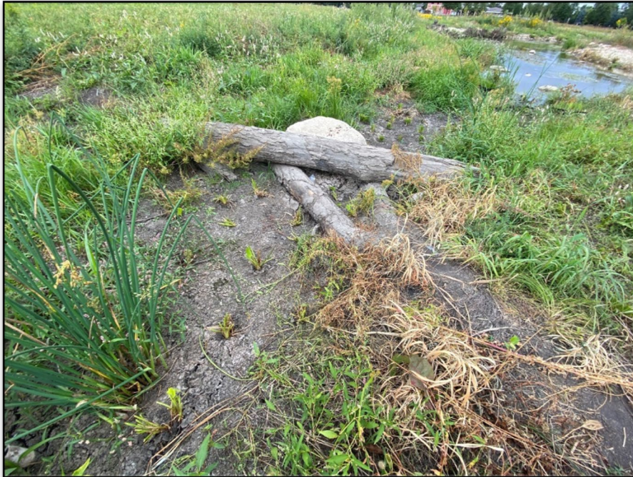
Plate 31. Looking downstream at a constructed oxbow in the previous streambed location. Wood harvested onsite and stabilized in place with boulders. Plugs are visible in the foreground during abnormally low flow conditions.
