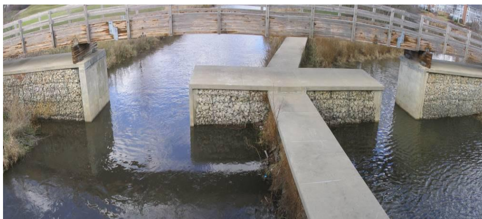
East Branch structure is 20 feet wide while the Prentiss Creek structure is 10 feet wide.
